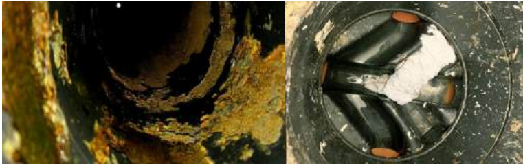
Figure 7.1 The condition inside of the pipeline: Corrosion and blockages
